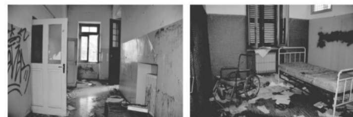
Fig. 7 L'Aquila, former asylum of Collemaggio. Abandonment and degradation in one of the corridors of the pavilion for the agitated sick. (photo: Martina Nardis, 2018)
