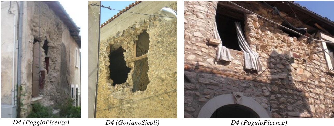
Fig. 9. Delamination of external and/or internal leaves of three-leaf masonry walls
