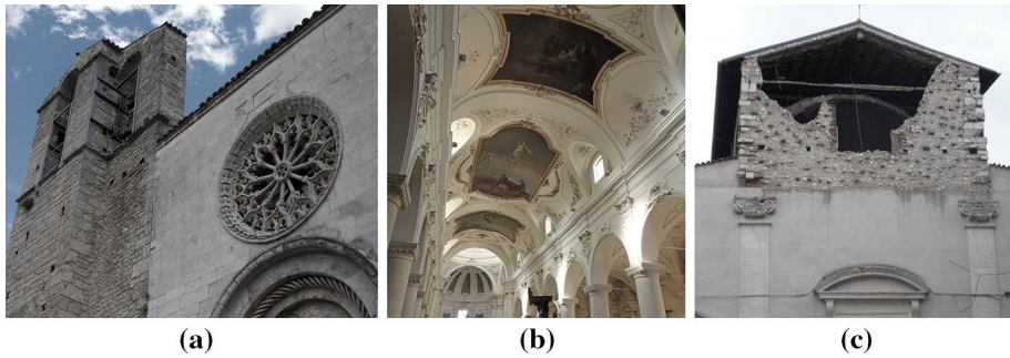
Fig. 23 Large openings in the façade of St. Maria Assunta church in Assergi [SAN; AQ] (a) ; thrusting vaults in St. Panfilo cathedral in Sulmona [SPA; SU-VA] (b) ; R.C. roof in St. Biagio d'Ameritum church in L'Aquila [SBM; AQ] (c)
