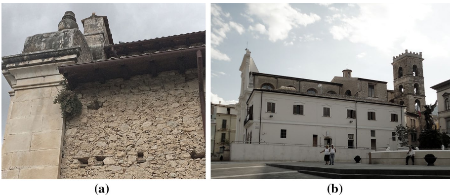
Fig. 20 Lateral wall-roof connection in S. Maria Extra Moenia church in Petogna [SMX; AQ] (a); building leaned on lateral walls in S. Maria Maggiore church in Raiano [SMM; SU-VA] (b)
