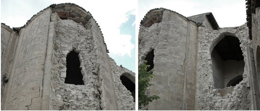
Fig. 13 Collapse mechanism detected in the apse of St. Eusanio Martire church in S. Eusanio Forconese [AQ]
