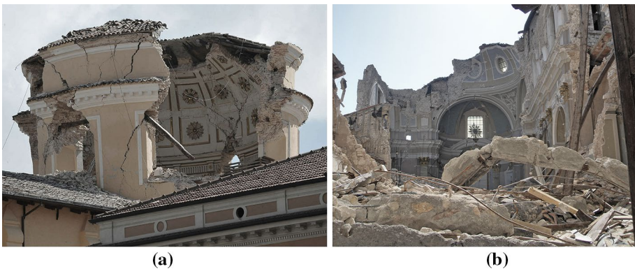
Fig. 14 Wooden ties in the dome of St. Maria of Suffrage in L'Aquila [AQ] (a); rigid ring beams in St. Maria of Paganica in L'Aquila [AQ] (b)
