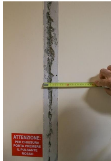
b) Insufficient expansion joints
