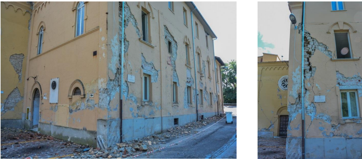
Fig. 2.2 – Amatrice hospital: damage to the masonry building and annexed church.
