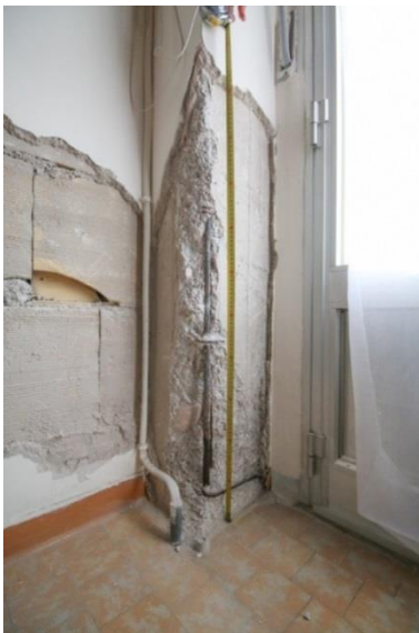
Fig 4.1.3 - a) Spalled concrete of a column
