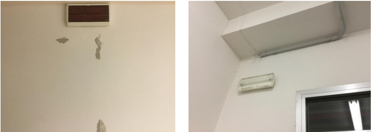
Fig. 4.2.5. Non-structural damage observed along the partitions and the infills of the upper floors of building block D.
