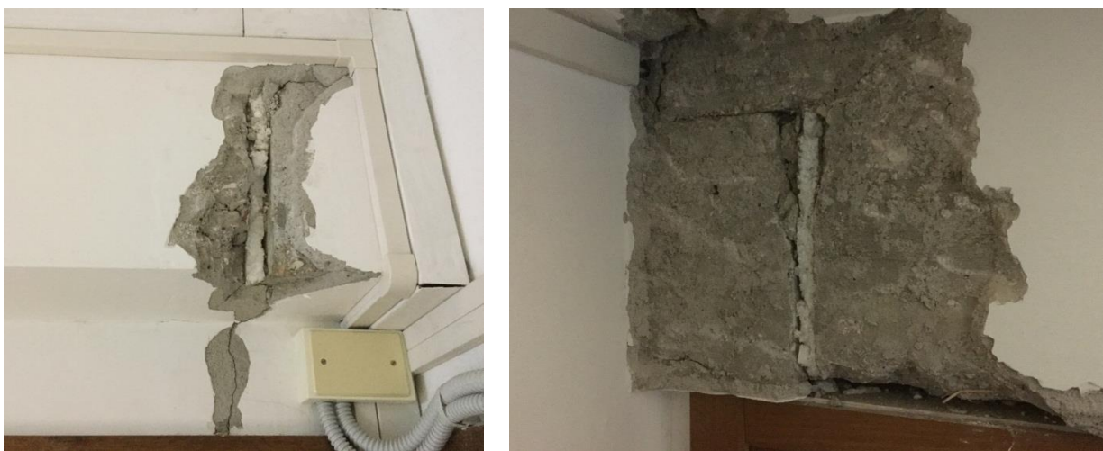
Fig. 4.2.6. Damage observed at the location of the Gerber saddle between building Blocks C and D.
