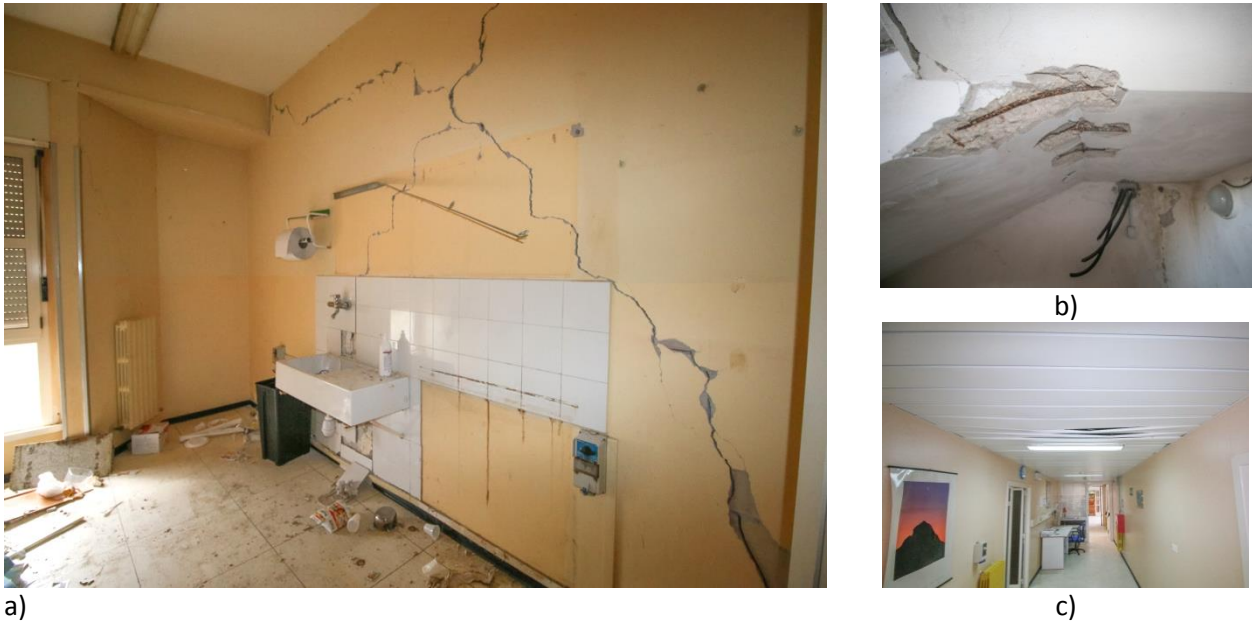
Fig. 2.4 – Amandola hospital, damage to a) partitions, b) stairs and c) suspended ceilings.
