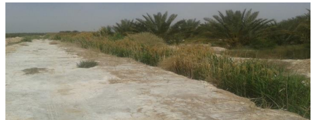
Figure 4 Drainage ditches infested by vegetation (oasis 3). It shows the problem of waterlogging because of poor or defective drainage. Here, the salinity is excessive and the alkalinity is high.
