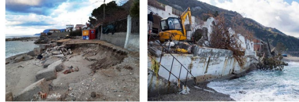
Figure 6. Favazzina: destroyed beach and damaged houses due to the sea storm of 23 December 2019.
