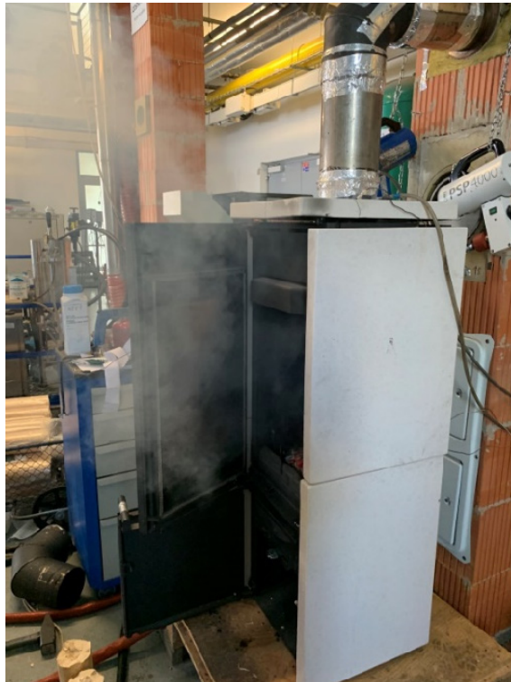
Figure 6: Accumulated flue gas rolls out of the combustion chamber.
