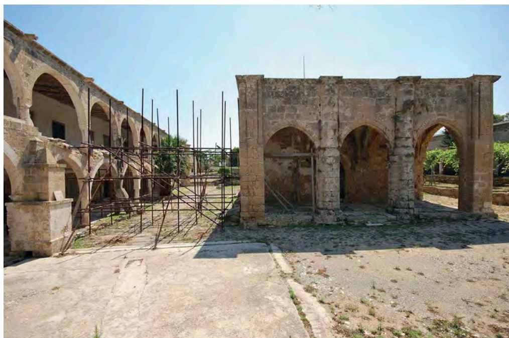
Figure 4. The scaffolding is holding in place the leaning column, urgent intervention is required (photo: A. Camiz, 2014).
