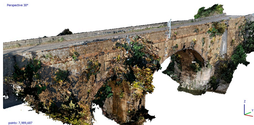
Figure 8. Three-dimensional point cloud of San Cono bridge (visualization in Agisoft Metashape software).
