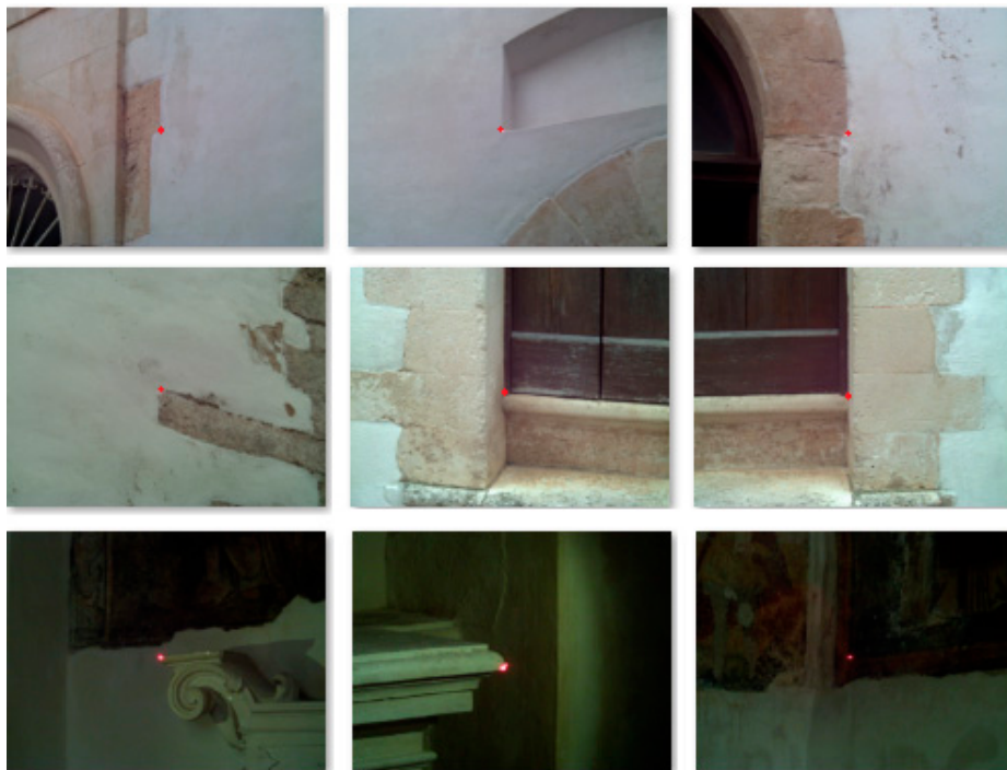
Figure 4. Images of some ground control points used for the georeferencing of the point cloud.
