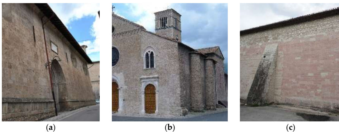
Figure 19. Examples of different types of buttresses: (a) buttresses obtained by widening outwards the masonry walls at the ground level in S. Maria Argentea church, Norcia; (b) circular buttresses inserted after the expansion of San Francesco Church, Terni; (c) classic “triangular” buttresses in San Agostino Church, Cascia.
