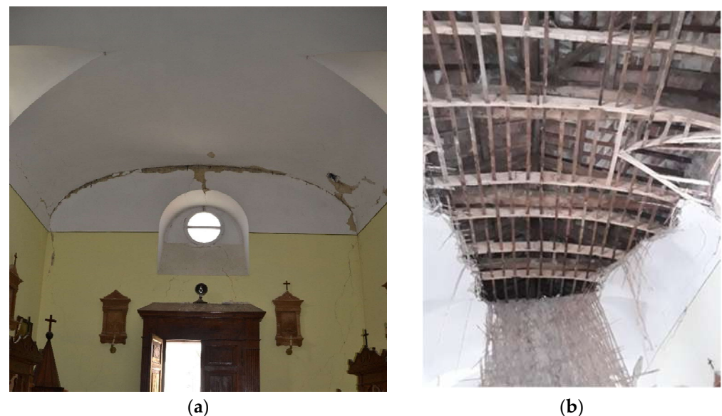
Figure 29. Internal view of the church of Santa Giusta in Amatrice: (a) lunette vault in “ camorcanna ” (September 2016); (b) collapse of the vault (January 2017).
