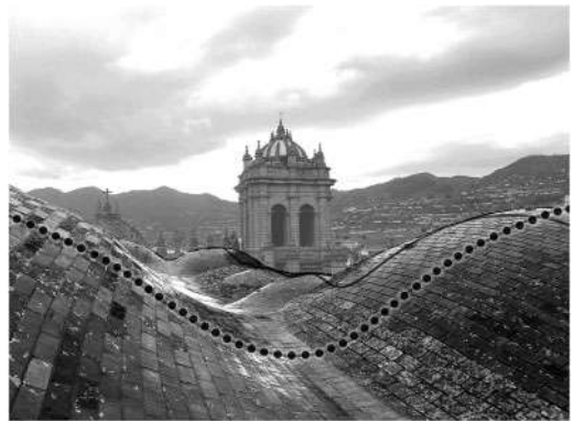
Figure 9. Cathedral of Cusco. The “flat roof” and the extrados of the vaults (the slope of the surface in evidence).
