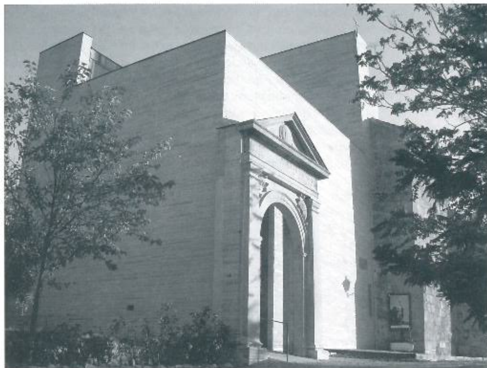
Fig. 3. Valdequeda, Madrid. San Lorenzo church. Detail of the Renaissance portal detached from the side entrance (Verazzo 2007).
