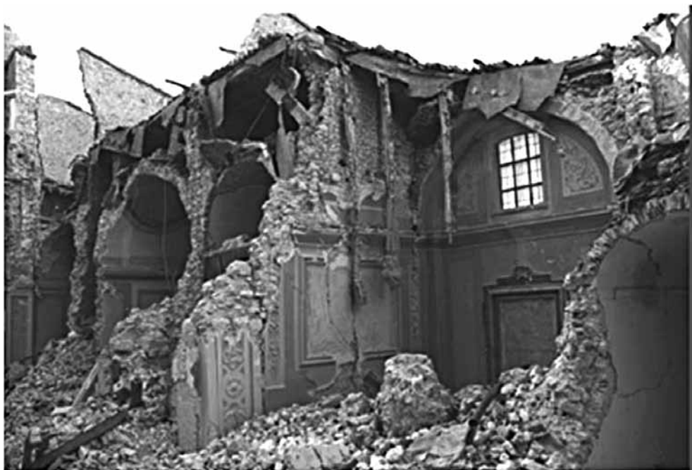
Fig. 21 - L'Aquila, S. Maria di Paganica, the interior after the 2009 earthquake (photo Author) .
