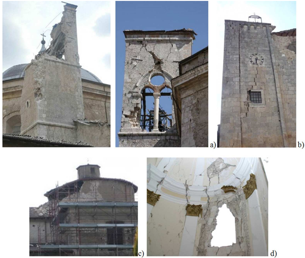
Figure 12. Diagonal cracks on wall after the 2009 seismic event. a) Bell tower of the St. Bernardino church (SBR) in L'Aquila and b) St.Eusanio Martire church (SEU) in Sant'Eusanio Forconese. Damages on the dome and the presbytery in c) St. Felice Martire church (SFM) in Poggio Picenze and d) St.Eusanio Martire church (SEU) in Sant'Eusanio Forconese. 83x70mm (300 x 300 DPI)
