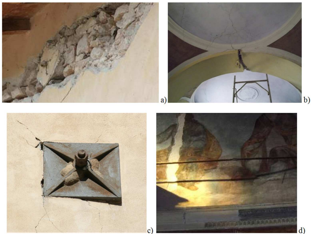
Figure 15. Effects of the 2009 seismic event on local elements of the studied churches: a) sliding cracks due to the reinforced concrete roof; b) damages on arches, c) punching phenomena and d) tie breaking.
