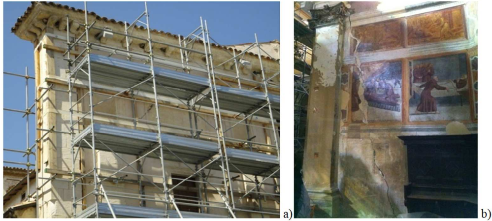
Figure 17. a) Top-corner overturning on St. Maria della Pace church in Capestrano and b) Apse overturning on St. Martino church in Gagliano Aterno. 86x39mm (300 x 300 DPI)
