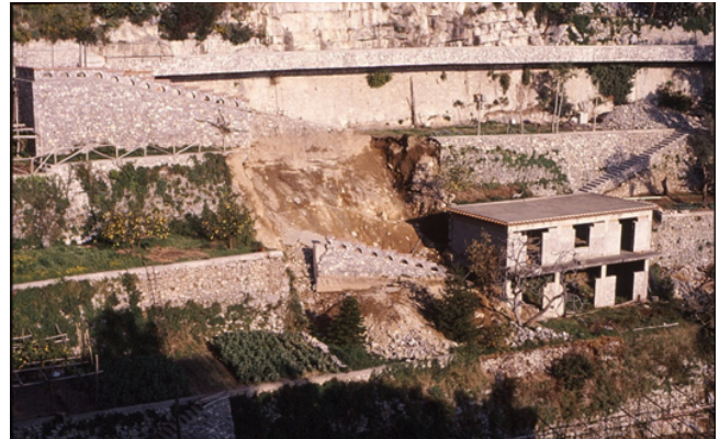
Fig. 1 – Typical landslide involving dry-stone walls on the Amalfi Coast
