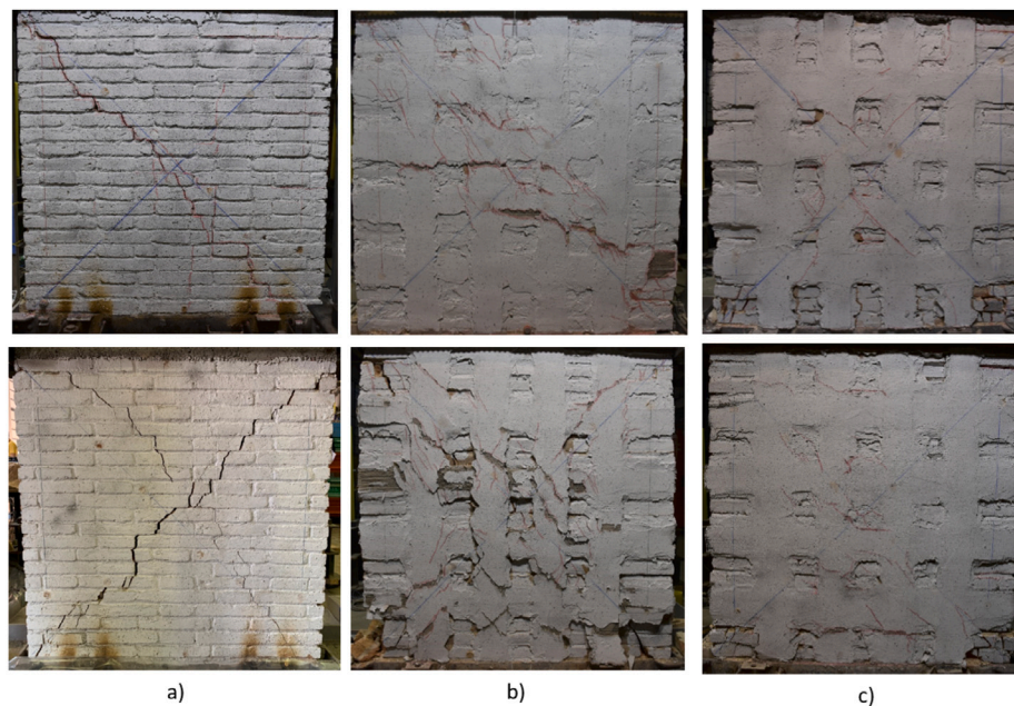
Fig. 6. Crack patterns at the end of the tests: (a) URM_1 (up) and URM_2 (down), (b) LDS_1 (up) and LDS_2 (down), (c) LDS-DL_1 (up) and LDS-DL_2 (down).
