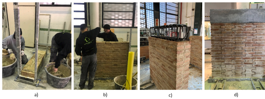
Fig. 1. Procedure for construction: (a) placing of the rulers for the construction, (b) construction of the wall in Flemish bond, (c) rebars placing for the concrete beam located on top of the specimen, (d) specimen finished and stored under laboratory conditions.
